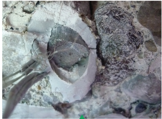
ETS installed bars (slip at the steel-epoxy adhesive interface)
