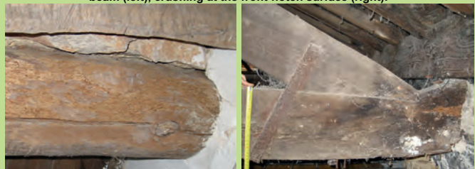
Figures 3 and 4: Floor beam damaged by insect attacks (left), Convent of the Christ in Tomar. Tie beam end decayed due to fungi (right), House in Porto.
