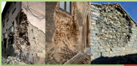
Local failures in masonry buildings 1 Fig. 1
