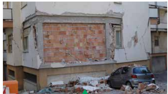
Failure of infill masonry in out-of-plane direction (L'Aquila, Italy).
