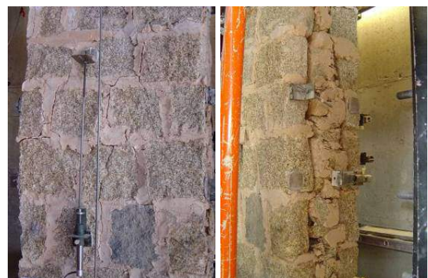
Figure 3 – Observed failure modes (plain walls).
