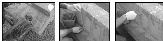
Opening the slits in the direction and with the desired depth. After the slit has been filled with the adhesive, the laminate is introduced. The adhesive in excess is removed. Fig. 2 – Main steps of the NSM technique for the shear strengthening.
