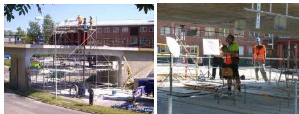
Fig. 3 – Crack detection in the failure test over Övik Bridge.
