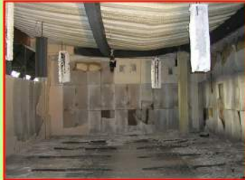
Compartment after fire
