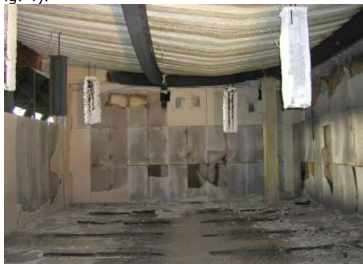
Fig 4 – Compartment after fire, residual deformation 925 mm, no local collapse of structure
