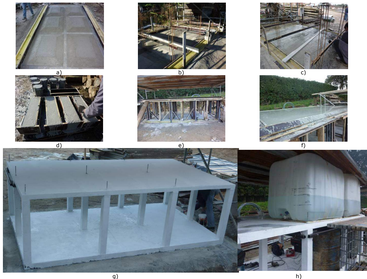
Fig. 1 The construction suspended slab prototype: (a) preparation of the foundation for the slab on grade; (b) Reinforcement of the columns; (c) casting the slab on grade (1st batch); (d) casting the SFRSCC specimens; (e) casting the columns (2nd batch); (f) casting the elevated slab; (g) general view of the prototype after has construction; (h) Water tanks loading corresponding to the serviceability limit states.
