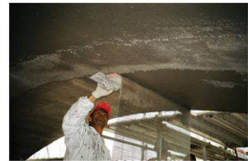
Strengthening of a masonry arch with fiber reinforced mortars. Courtesy of Ruredil S.p.A. (Taken from http://www.structuremag.org )
