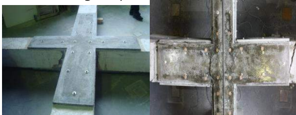
Fig. 7 Beam column joint before and after test.
