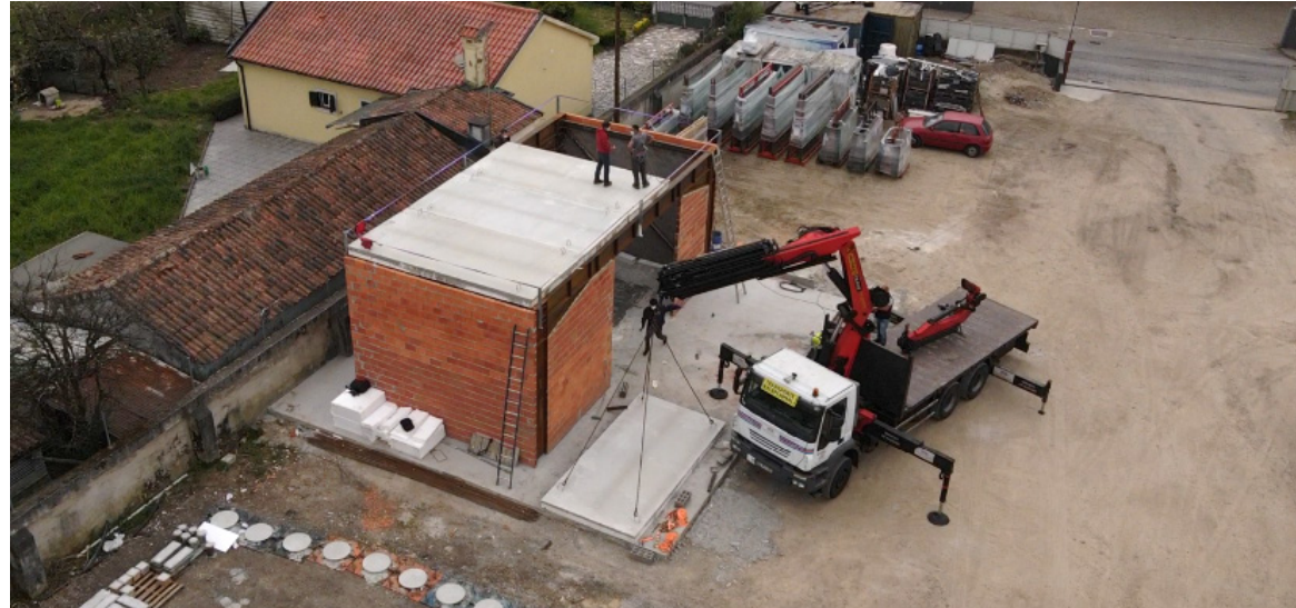
Building a real scale facility with a pavement made by PreSlabTec slab modules.
